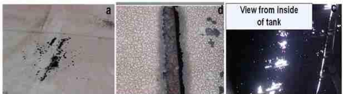
FIGURE 2. Examples of pitting (a-c) and crevice (d) corrosion on the tanks top that had coating for protection from corrosion
