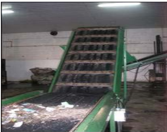
Figure 1 - USW treatment plant
