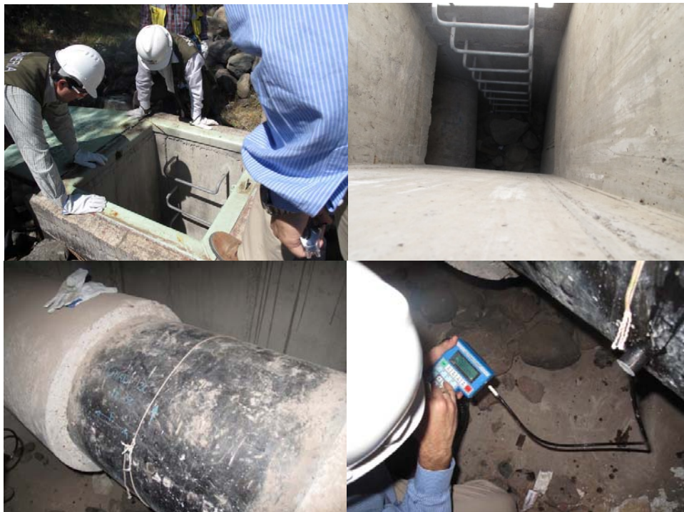
Figure 3 - buried enclosure for an existent pipeline
