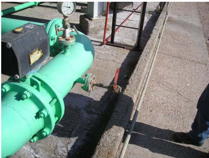
Figure 2-Valves show corrosion problems
